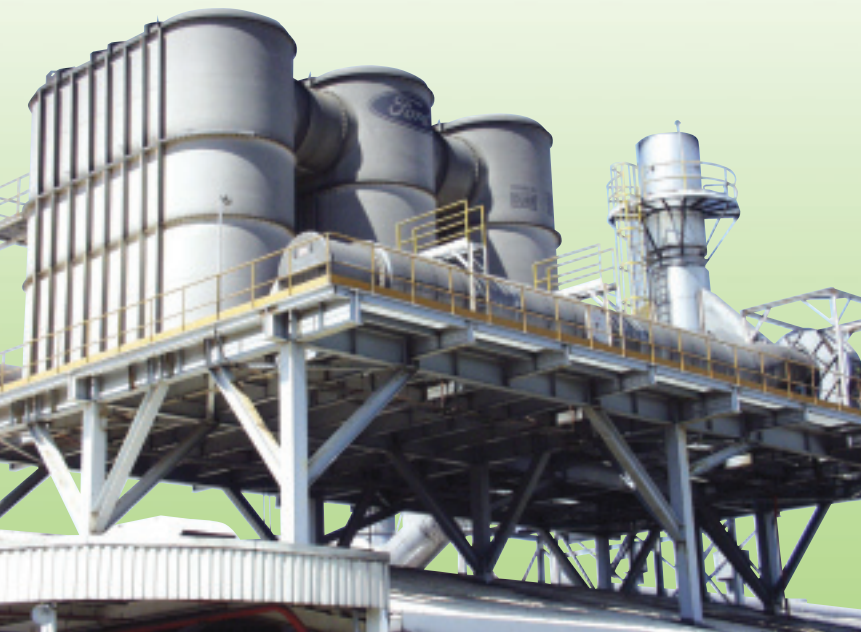
Air pollution prevention equipment— RTO
