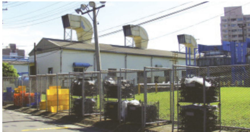
Sound insulation facility is installed in the air compressor room to prevent noise from disturbing nearby communities
